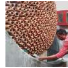
This Innovative Cooling Installation Fights Soaring Temperatures in New Delhi
